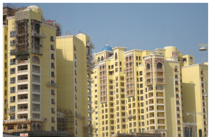
Photo 6: More Dubai stucco. Concrete frame, masonry backup wall has direct-applied exterior stucco. Thermal resistance is nominally R-8.
