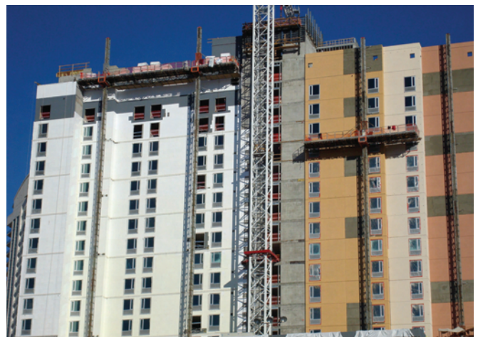
Photo 5: More Las Vegas stucco. Concrete frame, steel stud backup walls sheathed with paperless gypsum. Exterior insulation is EIFS. Thermal resistance is nominally R-20.
